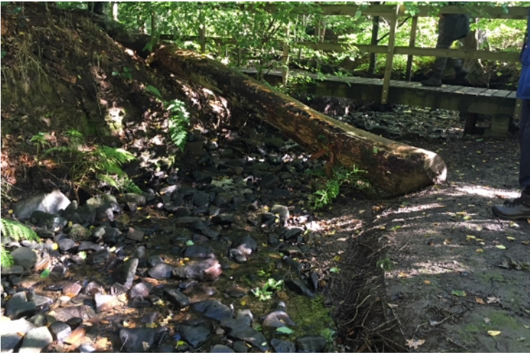
Fig 4. The bridge was moved about two cm down stream. The gabions were placed to the left of the bridge to reduce river bank erosion.
