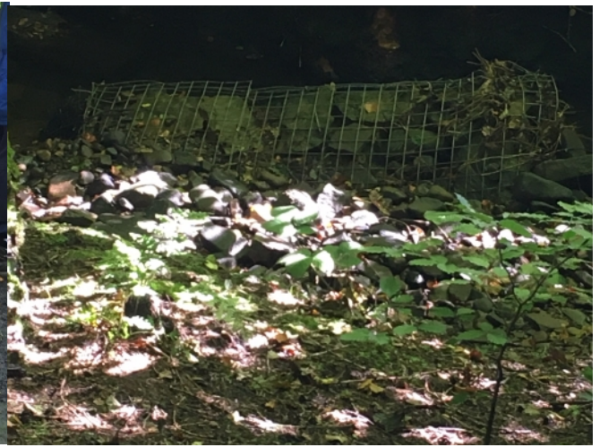
Fig 5. The gabion (it is about two meters long) that remained intact. We found the mangled remains of others farther downstream.
