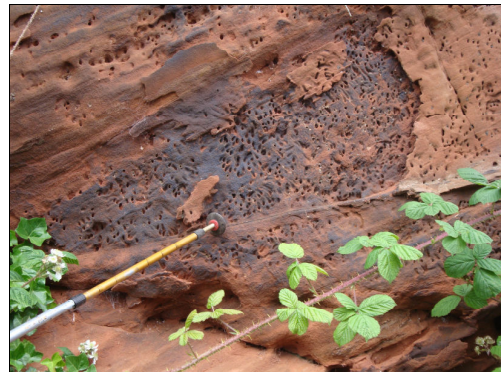
Bee Holes in the sandstones at Frodsham station (photo MDH)
