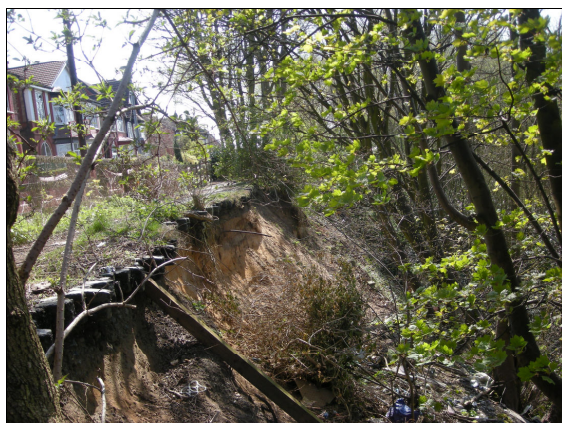
The Cliff landslide - note the precarious position of the houses ~ photo Marjorie Mosley
