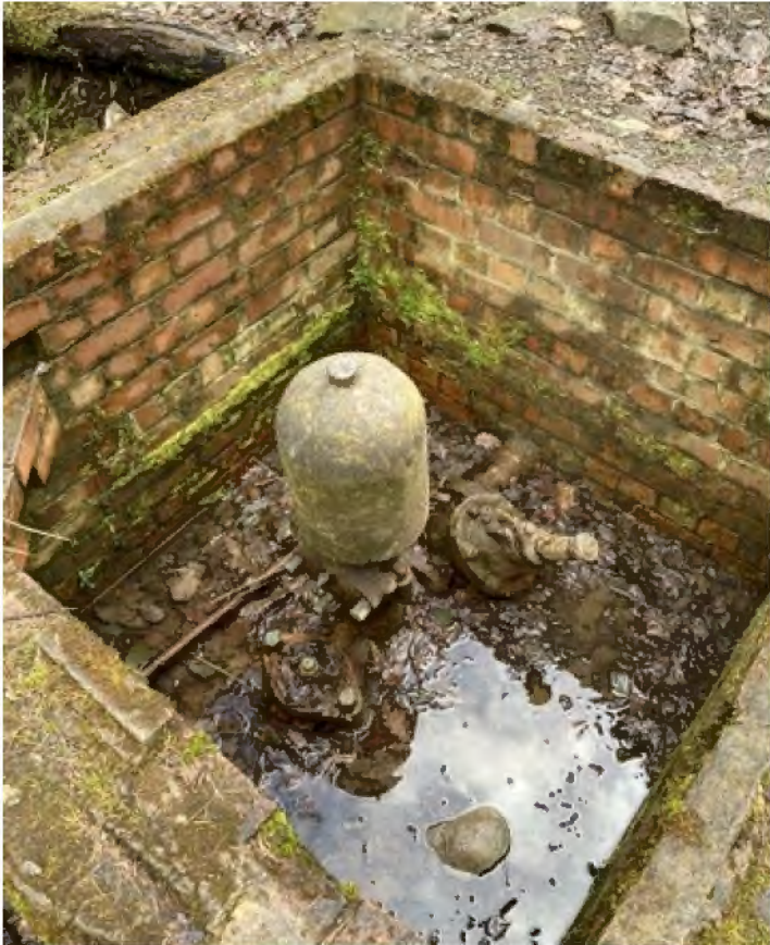
The Ram Pump, which uses the flow of the stream to pump water up to a storage facility.
