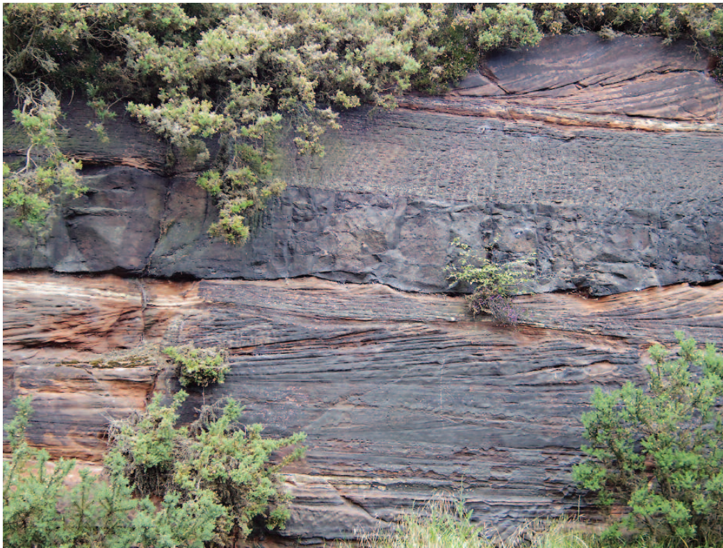
Fig. 2 Fault plane marked by the off-set creamy white bands. The fault has acted as a focal point for the penetration of groundwater which washes out the red, iron-rich stain in the rock.
