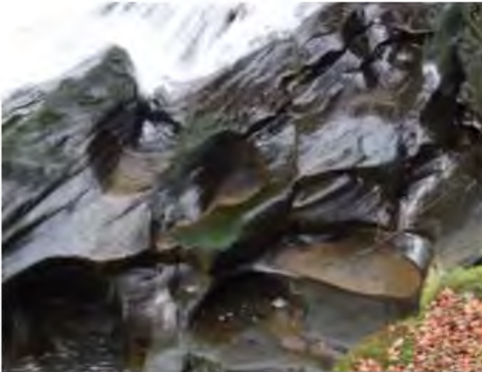
Figure 10: Potholes below the weir (Figure 9)
