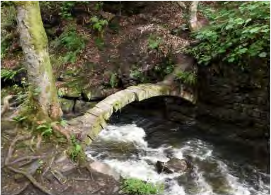
Figure 13: Arch over the Thrutch. Two arches once supported a building (see 10c).
