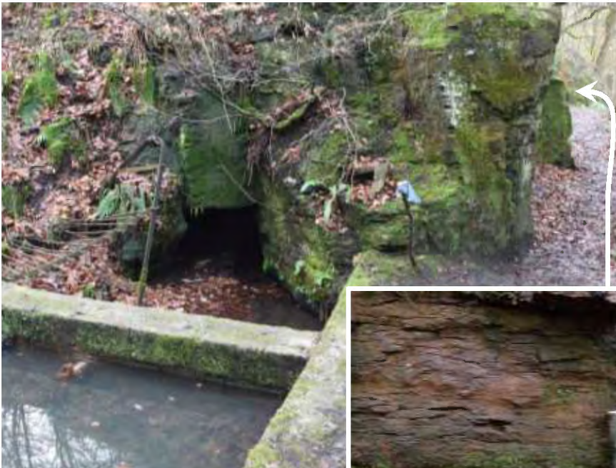
Figure 15: Water flowing from the leat on the left into the tunnel on the right. Inset bottom right: shales – see Location 12
