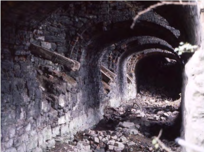
Fig 10: Remains of the wooden chutes used to transfer quicklime directly from the Bellman kilns to railway trucks
