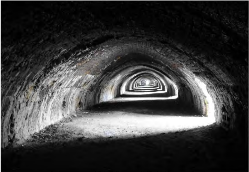
Fig 16: View down the tunnel on one side of the Hoffmann kiln at Langcliffe, near Settle
