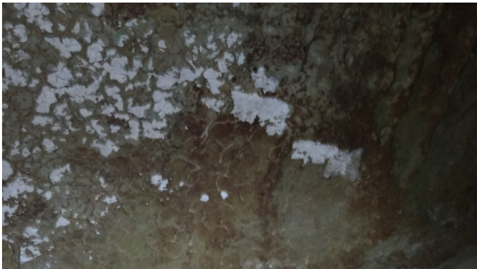
Desiccation cracks picked out by a lighter mineral
